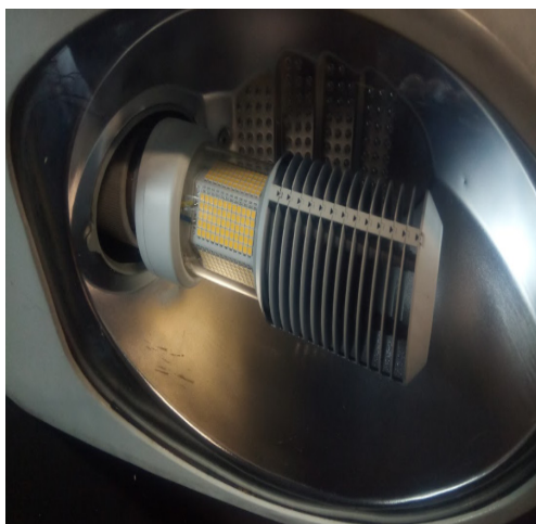
Figure 4. LED lamp in 150W HPSV light fixture
