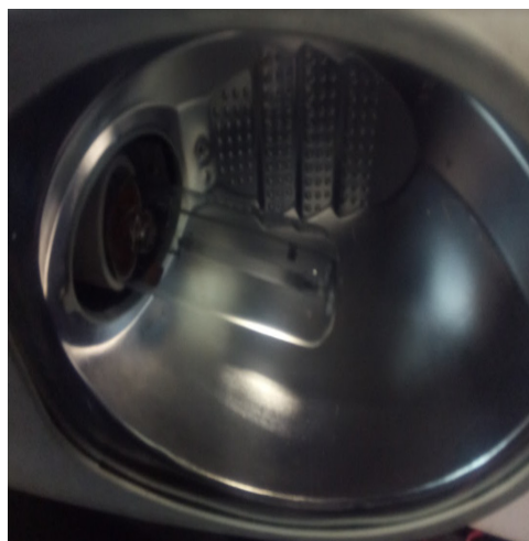
Figure 5. 150W HPSV lamp inside 150W HPSV light fixture
